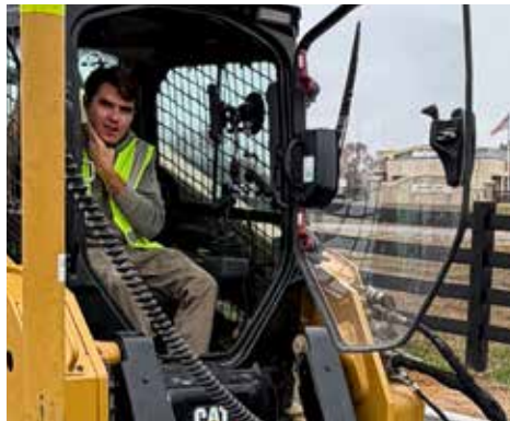
Sam Snow, Jim Smith Contracting at new casino in Calvert City, KY
