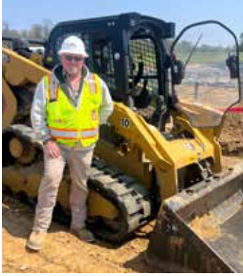
Robert Jones Jr., White Construction at Duff Solar Farm
