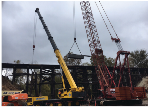
Sterett Crane and Marshall Crane on the Canadian National Railroad bridge replacement in Graves County, Kentucky.
