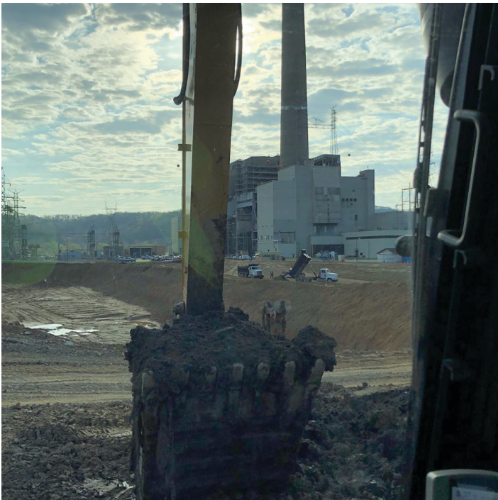
T.J. Moore on the Hoe for Entact loading trucks at AEP Big Sandy Plant
