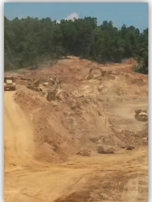
Jim Smith Contracting removing overburden at Warren Paving Quarry in Pinkneyville, KY.
