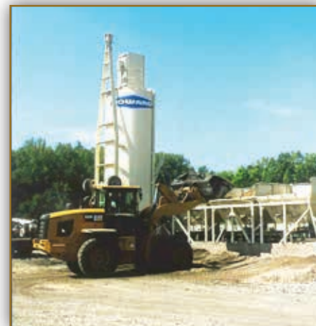
Howard Concrete Pumping at the McElroy Subdivisions project in Warrick County, IN.
